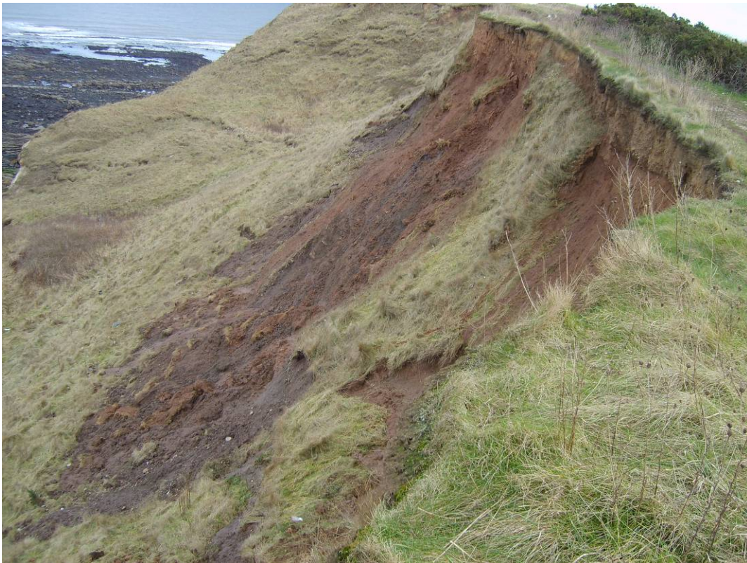
Plate 10 Slope erosion at Scalby Mills
