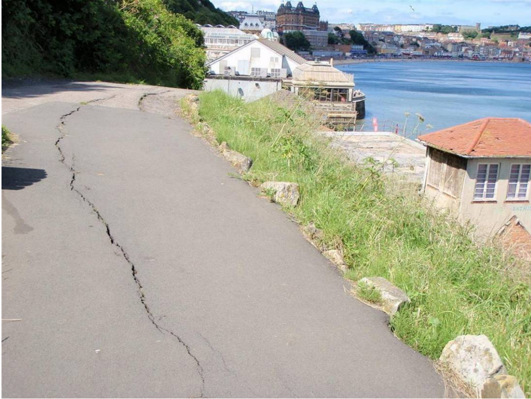
Plate 79 Scarborough South Cliff. Pavement cracks above the Clock Café (July 2008).
