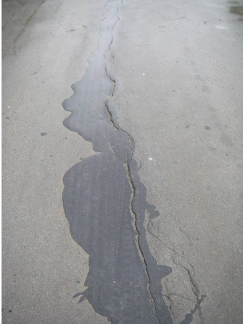
Plate 43 Site view of repair to tension cracks in lower section of access road (12 th Jan 2010)
