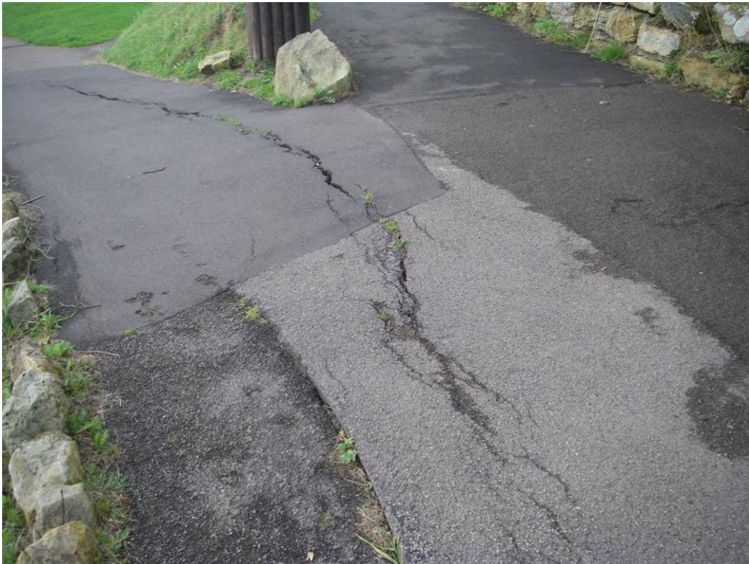
Plate 80 Scarborough South Cliff. Pavement cracks above the Clock Café (Sept 2008)
