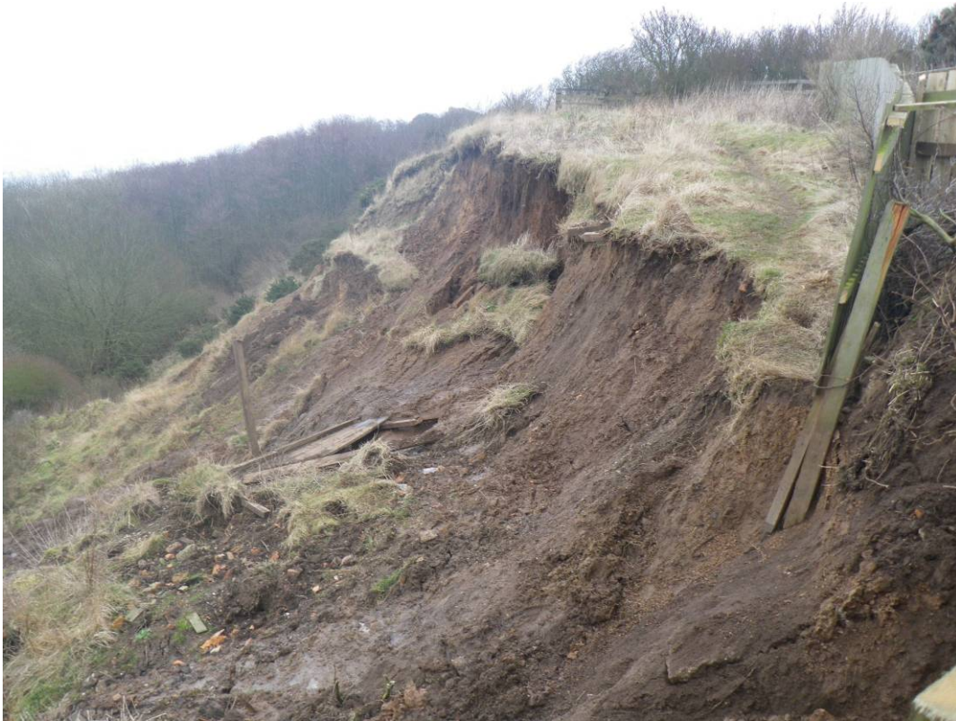
Plate 24 Slope failures on Cornelian Bay side of Knipe Point looking east (16 th March 2010)
