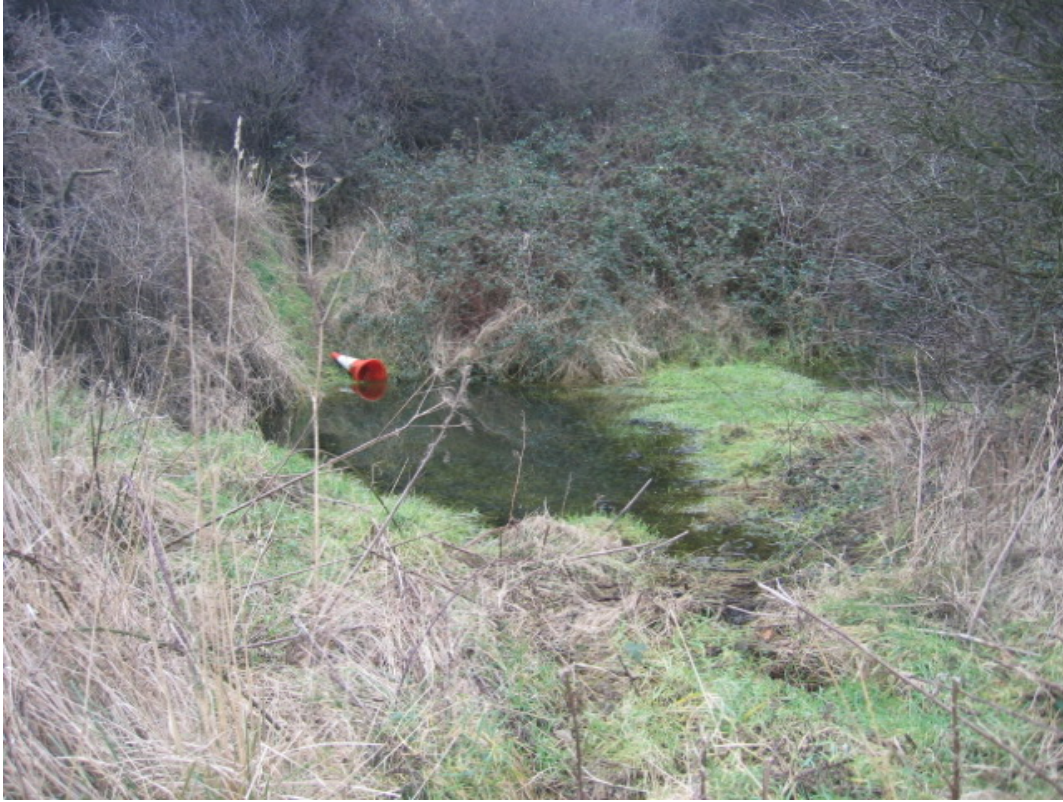
Plate 11 View of ponding water in mid-slope back rotated block area (January 2010).
