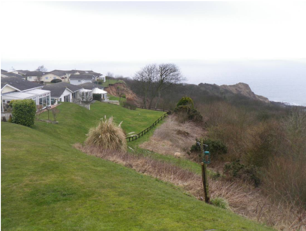
Plate 29 Cliff recession at Knipe Point Headland (8 th March 2010) looking east
