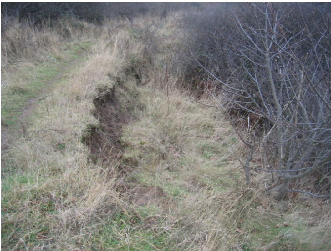
Plate 10 Site view of mid-slope back rotated block and surface tension crack development (January 2010).
