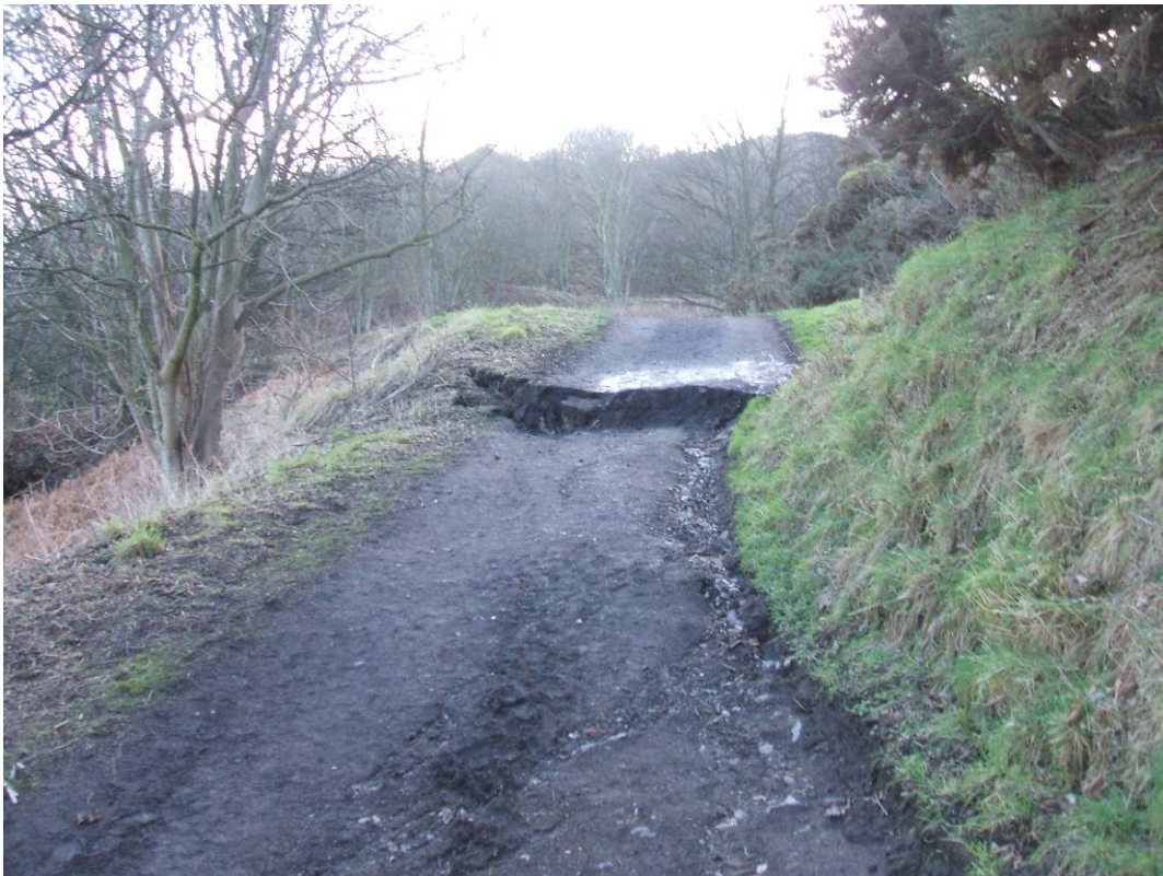
Plate 6 Slip in railway path at Sandsend
