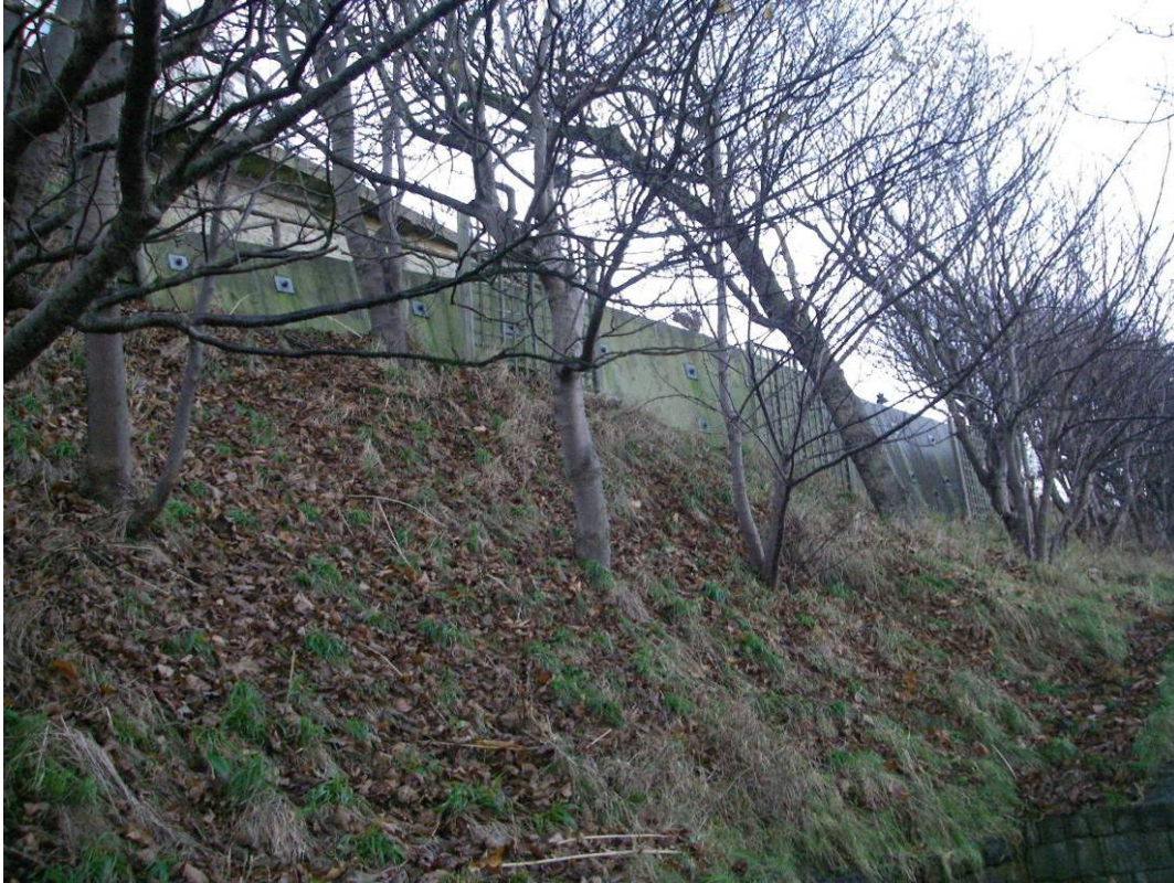
Plate 20 Site view of slope crest retaining walls at Prince of Wales Cliff.
