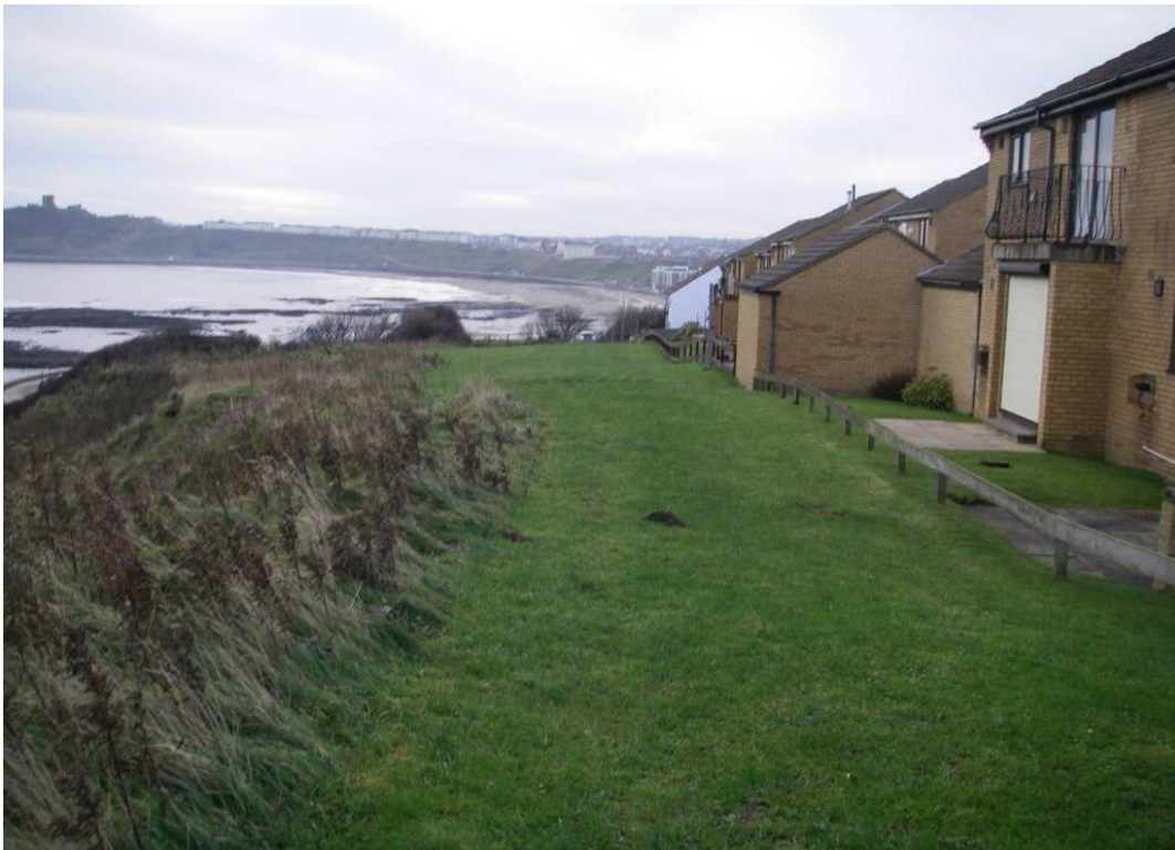
Plate 6 Site view looking south across Upper Plateau showing slope crest and residential properties.
