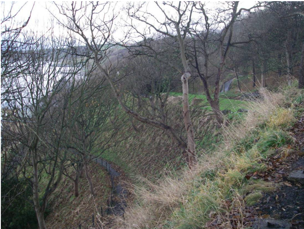
Plate 21 Site view looking south across Spa Cliff showing steep slope angles and bench-cut paths.
