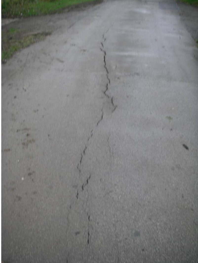
Plate 42 Site view of tension cracks in lower section of access road
