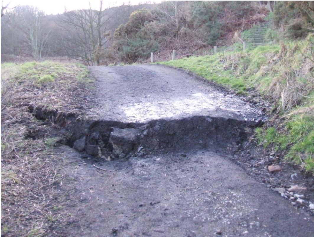
Plate 5 Slip in railway path at Sandsend
