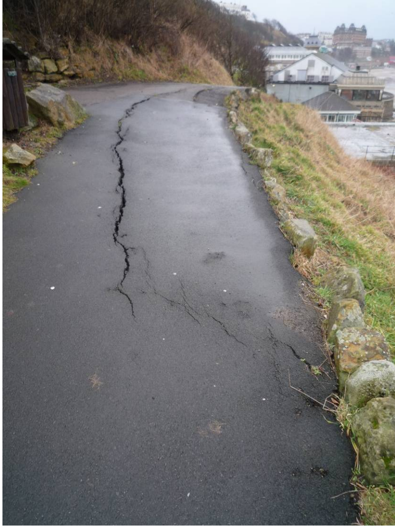
Plate 83 Scarborough South Cliff. Pavement cracks above the Clock Café (Jan. 2010).
