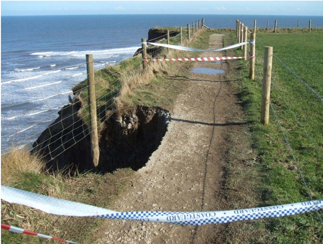
Plate 3 Cliff erosion at Saltwick
