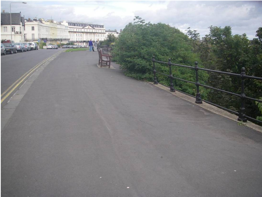
Plate 77 Scarborough South Cliff. Promenade showing signs of subsidence.
