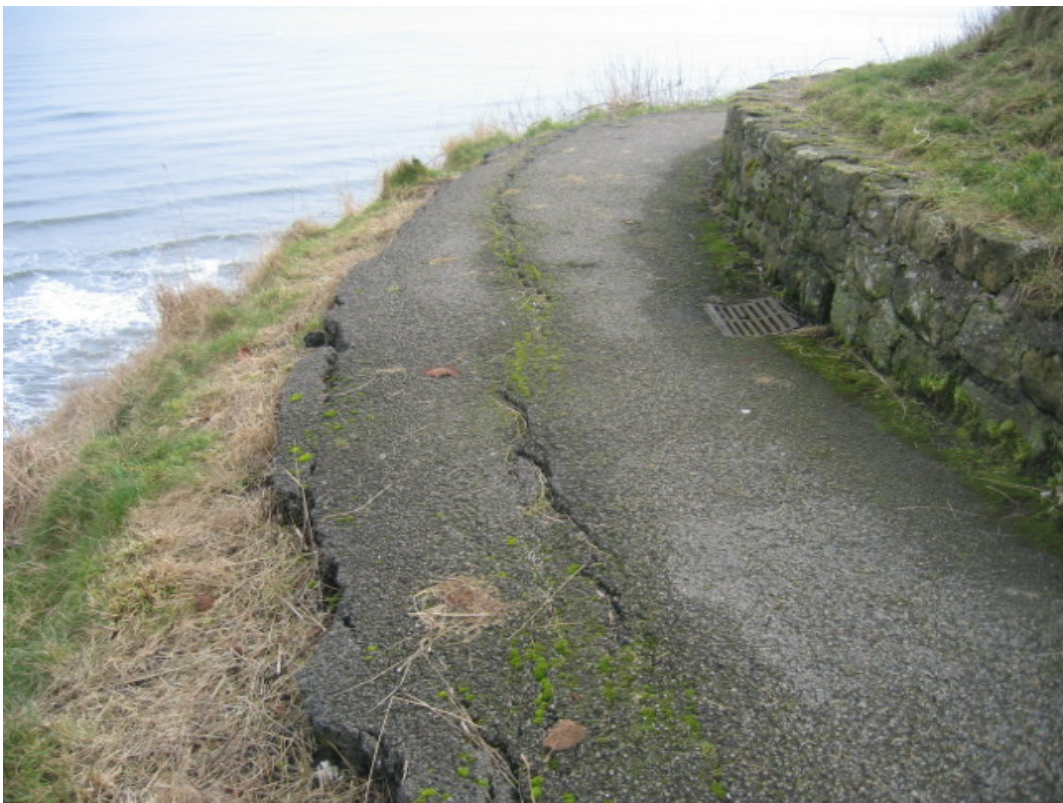
Plate 85 Footpath degradation around Holbeck Gardens.
