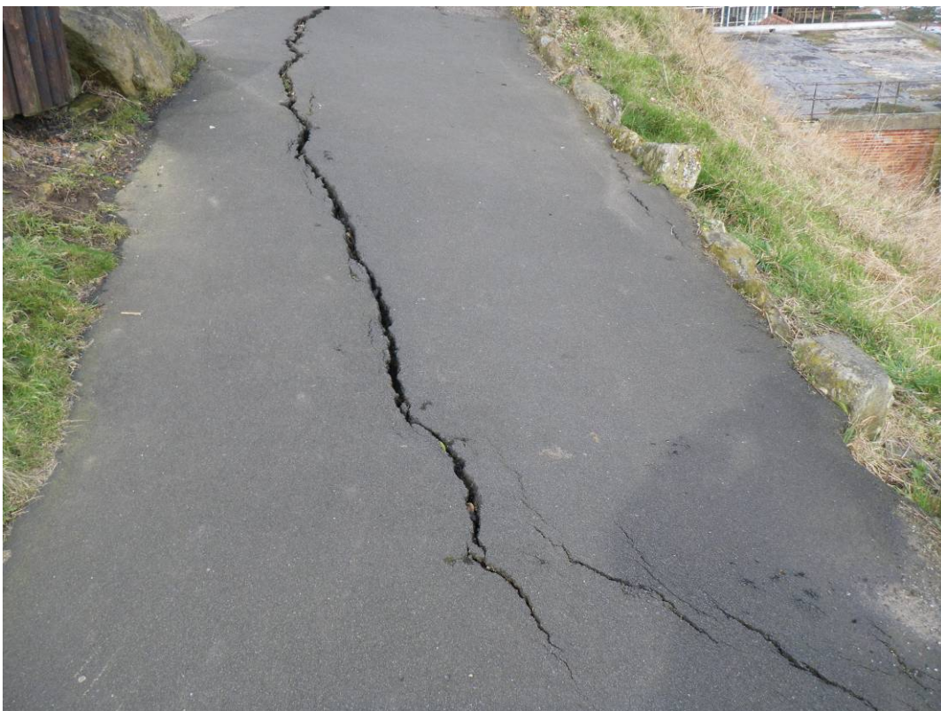
Plate 82 Scarborough South Cliff. Pavement cracks above the Clock Café (March. 2010)
