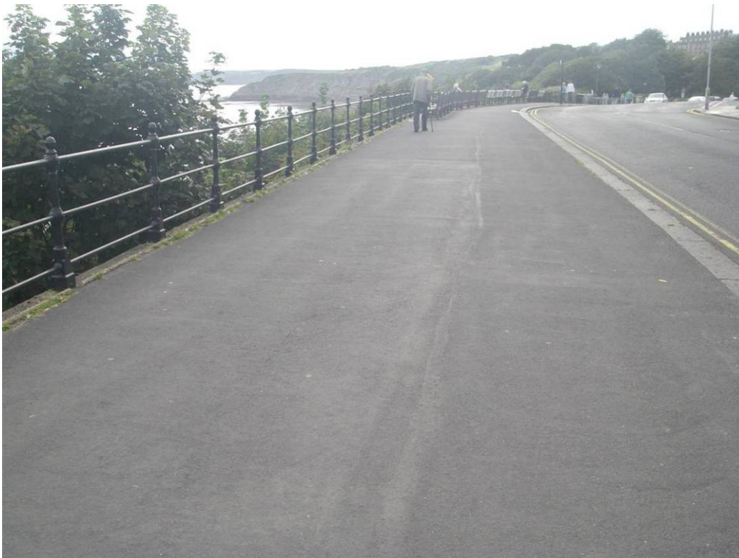
Plate 78 Scarborough South Cliff. Promenade showing signs of subsidence.
