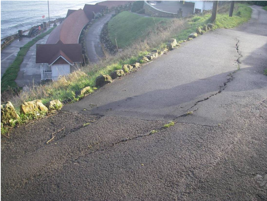
Plate 81 Scarborough South Cliff. Pavement cracks above the Clock Café (Dec 2008)
