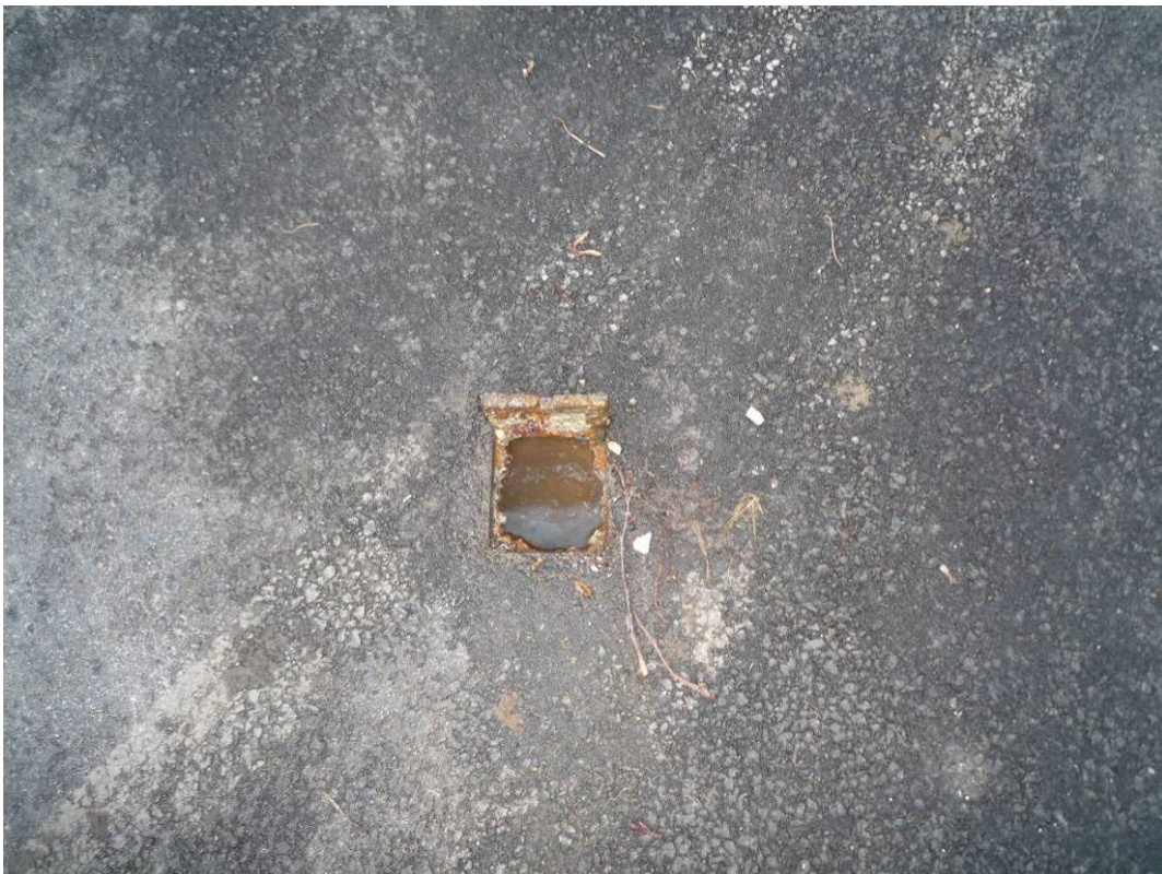
Plate 93 Filey Town BH02 (Flooded Headworks)
