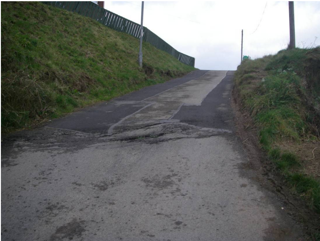
Plate 39 Site view of developing tension cracks and bulge in access road of Flat Cliffs.
